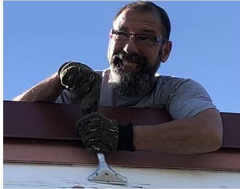
Alex Misiewicz enduring a hot tar roof on a very sunny day scraping away old paint from the fascia.
