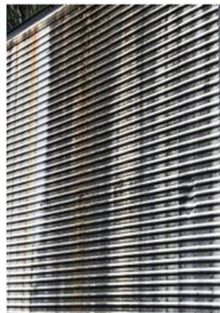
Vehicle exhaust, residue and corrosion on the storage trailer.
