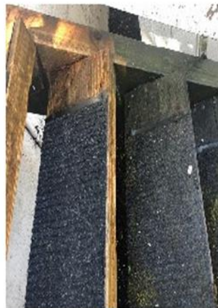
The tread on the right is covered with slimy moss and was discolored. The tread on the left is actually safe to walk on now.
