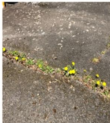
Dandelions, grass, weeds and moss growing on the asphalt and up through the cracks. Not anymore!
