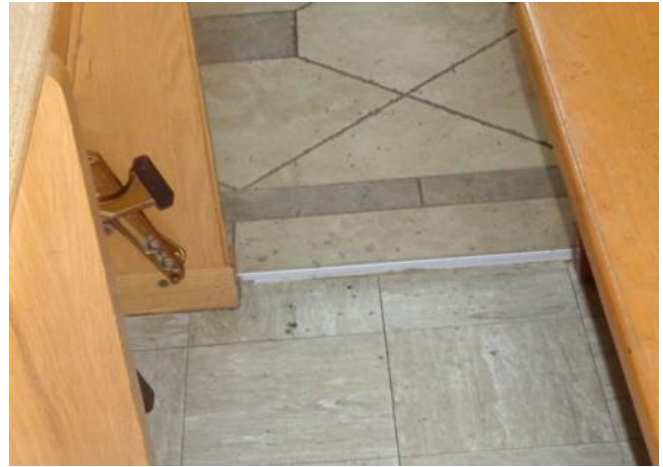
The existing flooring in the pew area is recessed about 2/4" below mosaic tile aisles. New laminate flooring with a plywood filler underneath would make it flush.
