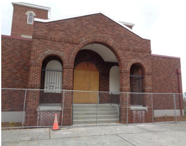
A large arched opening in the center of the Narthex entry overhang gable wall is where a lockable scissor security gate, still in procurement, will be installed. Temporary chainlink fencing with a lockable gate will remain in its place in order to keep the outside entry overhang area secure until the scissor door arrives. The original design called for an ornamental type double swinging gate, but the City of Tacoma would not allow it because the gates would have swing out onto the abutting city sidewalk area.
