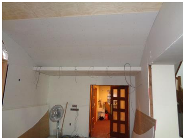
This is a photo of arched ceiling construction in the Narthex taking place in early September.
