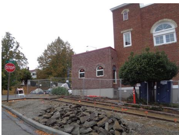
This photo shows the demo'd remnants of a sidewalk along 16th Street, and a new one behind the debris being prepped and ready to pour.
