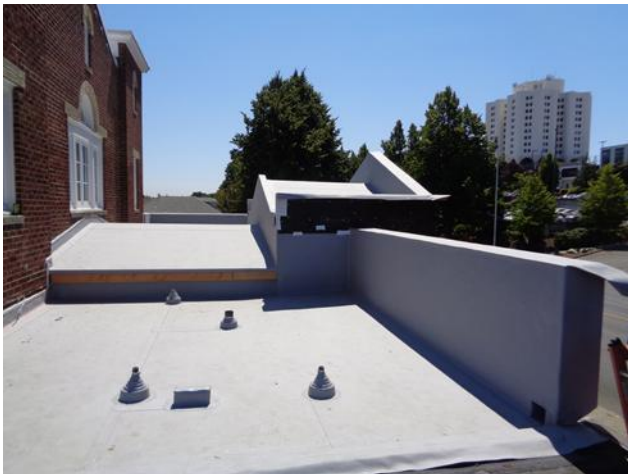
This is a photo of the new insulated roofing taken from the top of the Upper Hall over the sink area, looking from north to south towards 16th Street.
