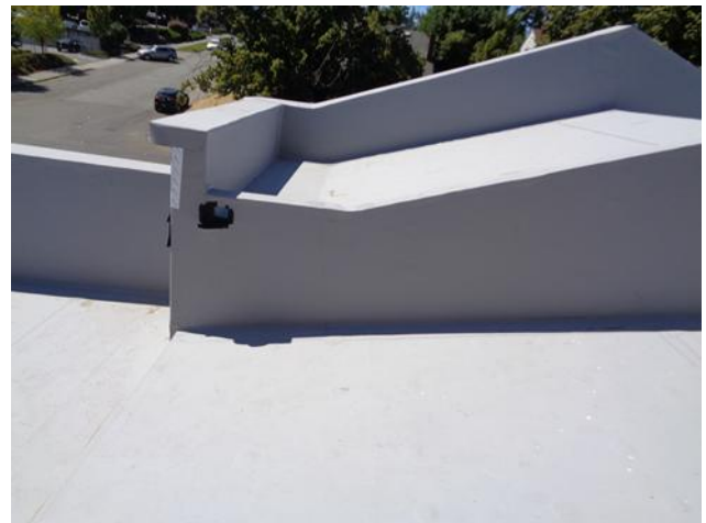
This is a photo of the back side of the Narthex entry, looking from east to west towards Yakima Avenue. Note that in both photos, all new roofing have drainage slopes built into their assemblies.
