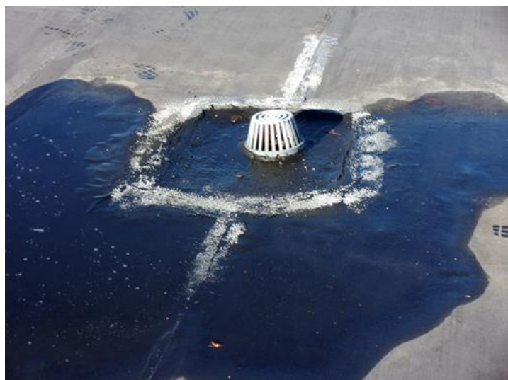
This is the Upper Hall roof drain near the center of a virtually no-slope roof. On rainy days a stagnate small lake will accumulate. A 10' x 10' liquid membrane preventative maintenance patch will be applied around the drain in dryer weather.
