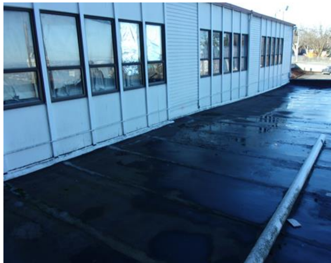
Above is a view of the Upper Hall bookstore and office areas taken from the Dining Hall roof deck. The scenery on the roof is less attractive in real life, especially when wet and puddling.
