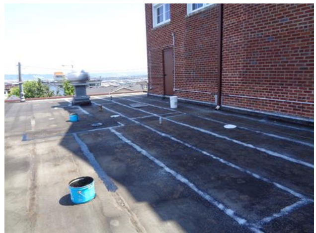
Above is the Dining Hall/Kitchen roof looking east. The light colored stripes consist of mastic with white granules on top, applied to roofing seams and other suspect areas as a preventive maintenance effort.
