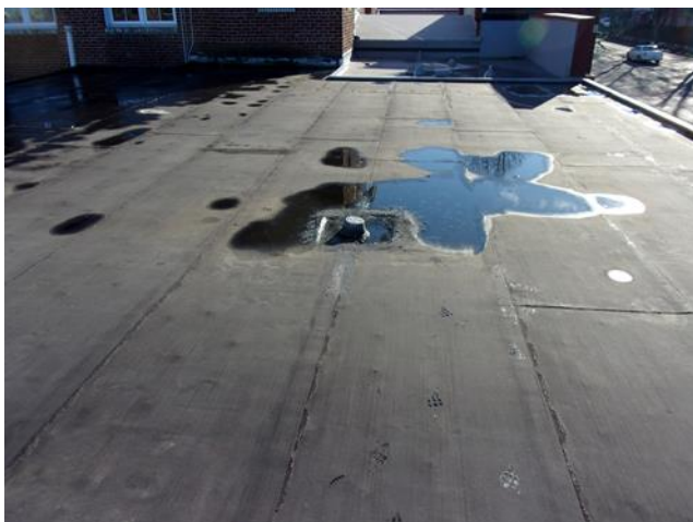
This is the roof drain area over the Upper Hall, shot on a sunny day a few months ago, looking north towards the Narthex. Note the standing water puddles that linger on a roof that has no slope built into it.
